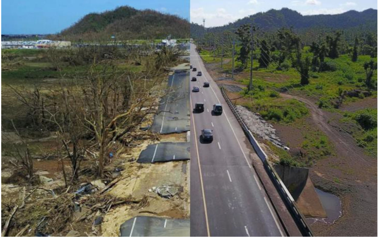
Splice of post-Maria damaged and repaired road and overhead lines in Toa Alta, west of San Juan. Source: Ricardo Arduengo/AFP/Getty Images 1
